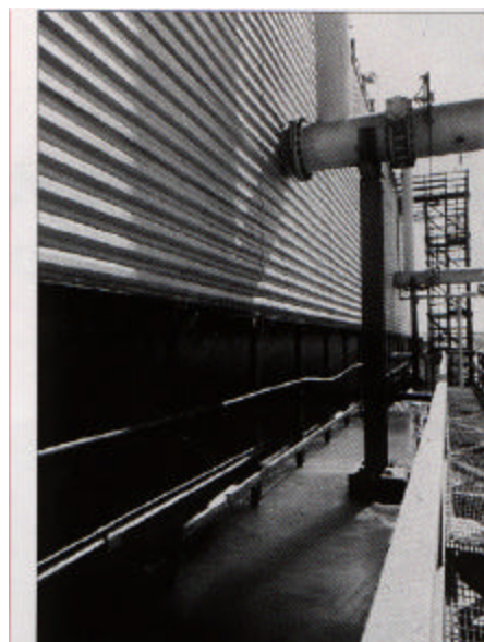
Using Redox control, the accurate oxidant level is now maintained, resulting in improved biological control and reduced potential for fouling and corrosion problems.
