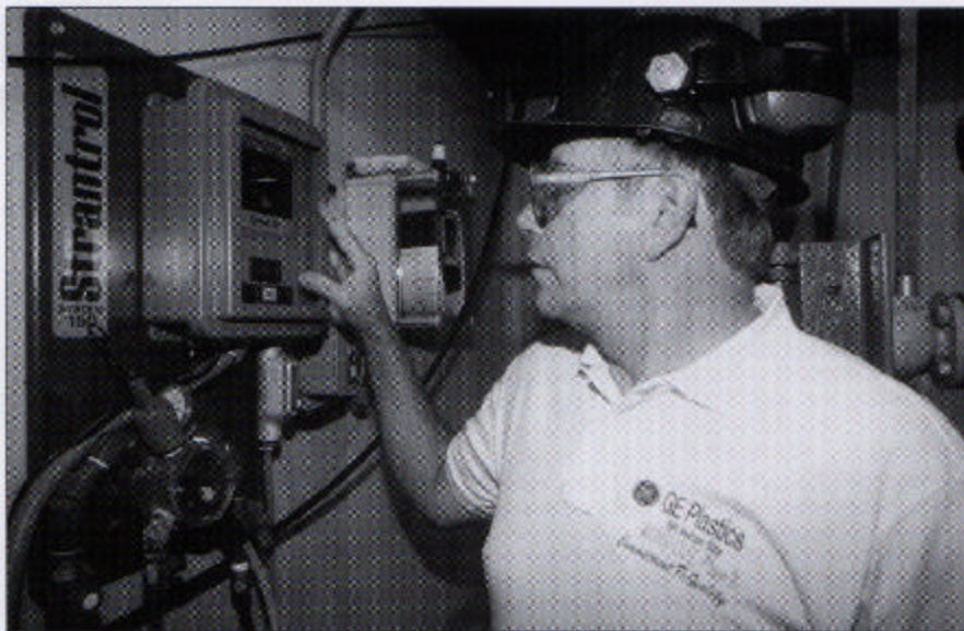
Don Ricketts, Lab Specialist at the GE Plastics plant, checks the current millivolt reading of the High Resolution Redox control system. The system constantly monitors the oxidant demand in the cooling tower's return water and automatically feeds the required amount of NaOCl to achieve and maintain system cleanliness.
