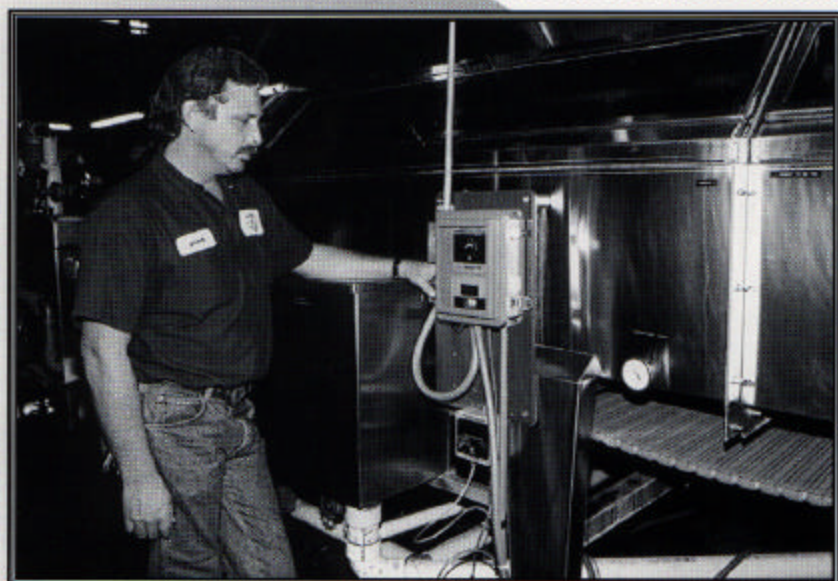
Maintenance Technician Jake Jeffries examines the pasteurizer's HRR-based chlorine controller from Stranco, Inc., Bradley, IL. Maintaining an HRR setpoint of 722 mV ensures a 2-3 ppm chlorine residual.
